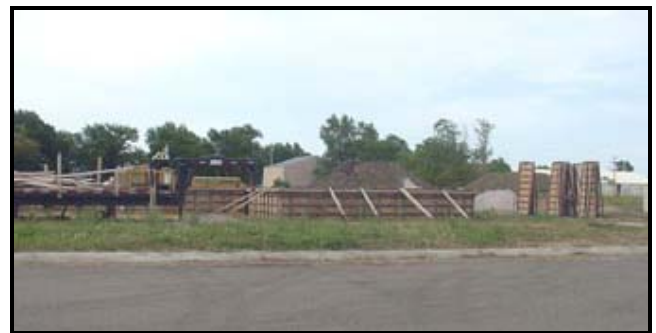
The foundation is being prepared for house placement at the White Lake sites.
